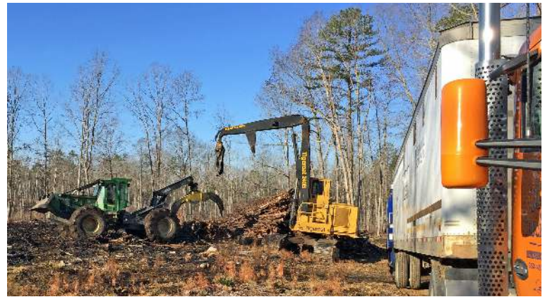
Proper communication and spacing are key to log deck safety.
